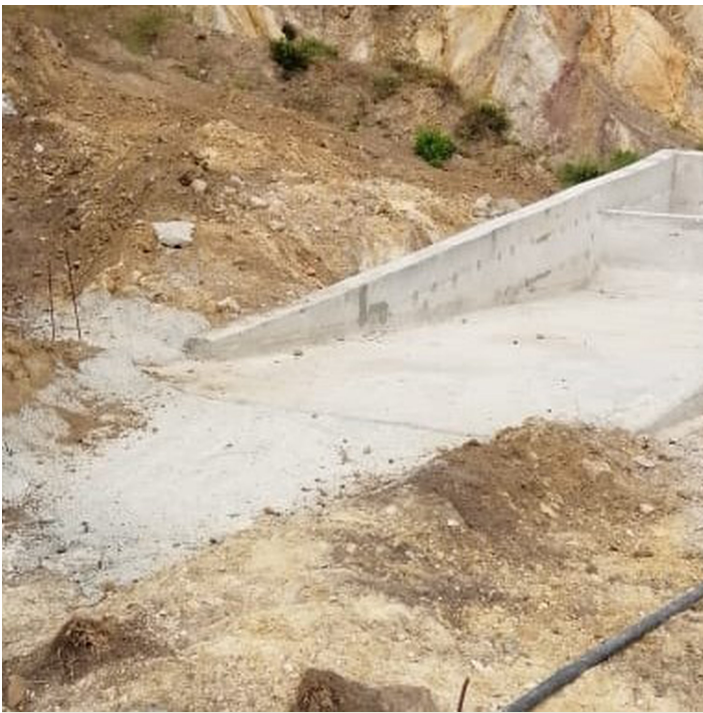
Sedimentation trap, located above the pond to settle the sediment transported by the runoff water
