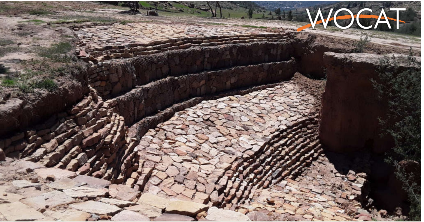
Gully head is constructed at the head of a gully using stones to discourage the gully from expanding further in length thereby stabilising the gully. (Koetlisi Koetlisi)
