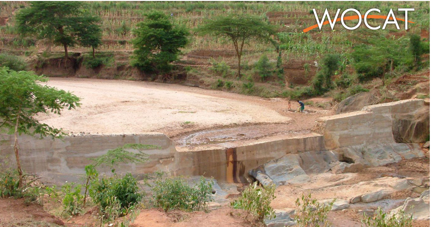
An example of a mature sand dam in the Nzyaa Muysio valley (Simon Maddrell (Excellent Development, 59 Market Building, 195 High Street, Brentford, UK))
