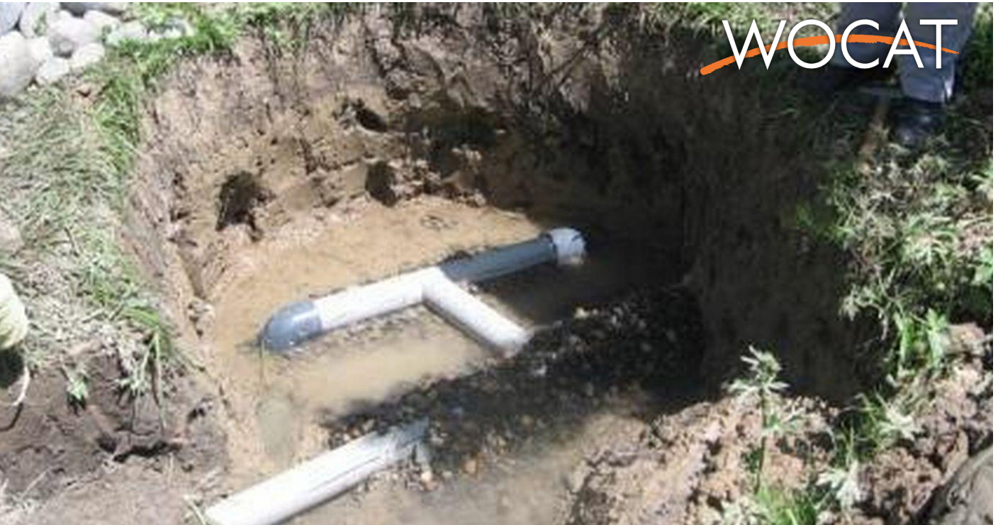
Perforated pipes placed upon a gravel bed to stop them from becoming clogged. (Giuseppe Bonaty (CESVI))
