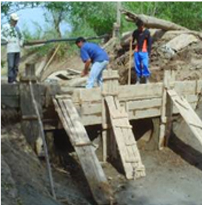
Construction of small hydraulic structures in the head of the channel (Eshchanov R.A.)
