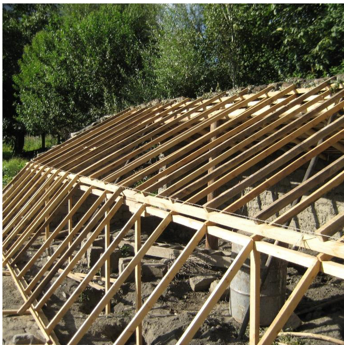
South-facing side of a solar greenhouse during construction process before the cellophane layer was put in place (MSDSP Khorog)
