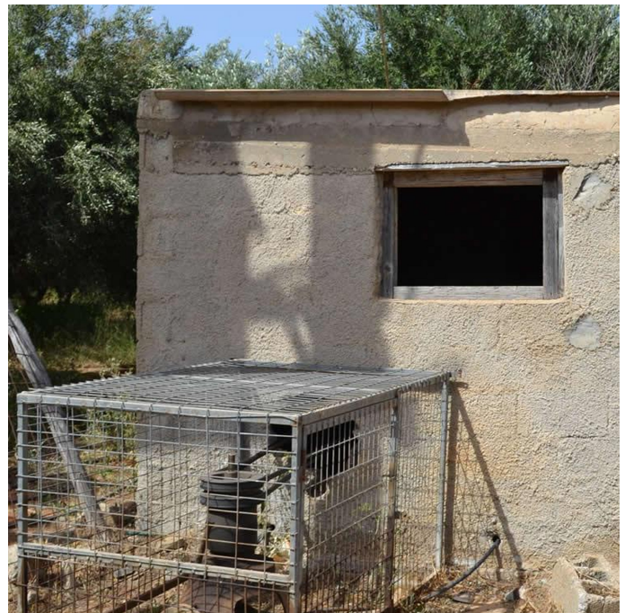
Traditional 'Pomona' type turbine water pump and pumping station (I. Daliakopoulos)
