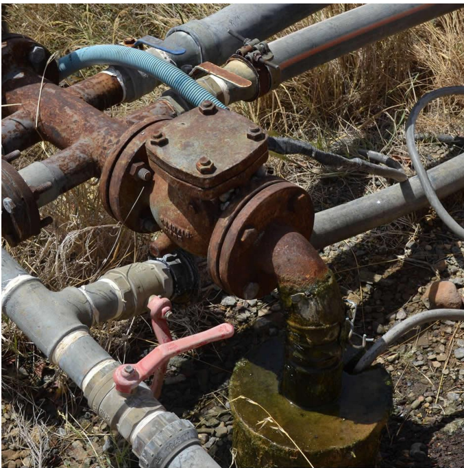
Submersible pump and distribution network (I. Daliakopoulos)
