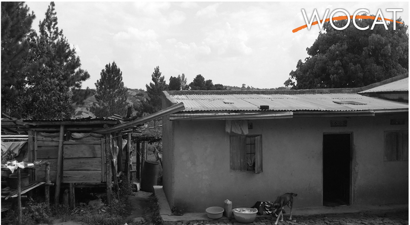
Front view of the rain water harvest reservoir structure and the home roof top. (Aine Amon)
