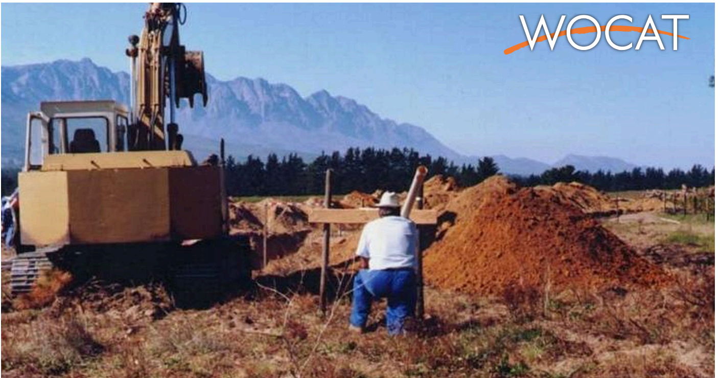
Drainage (Hans King)
