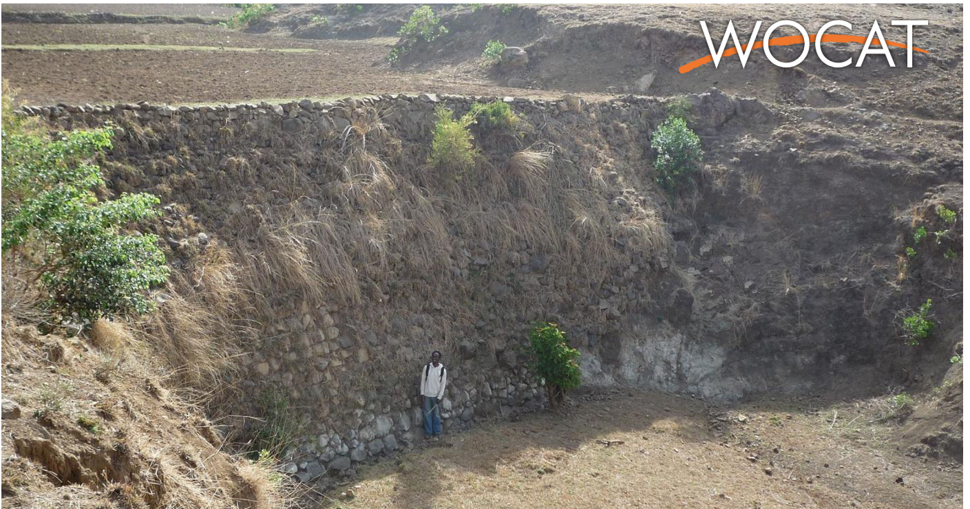
A large stone check dam across a deep gully. (Simon Bach (CDE, Bern, Switzerland))
