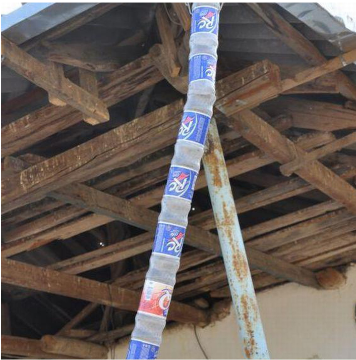
The plastic pipe running from the roof to the concrete tank. (S. Stevenson (Camp kuhiston))
