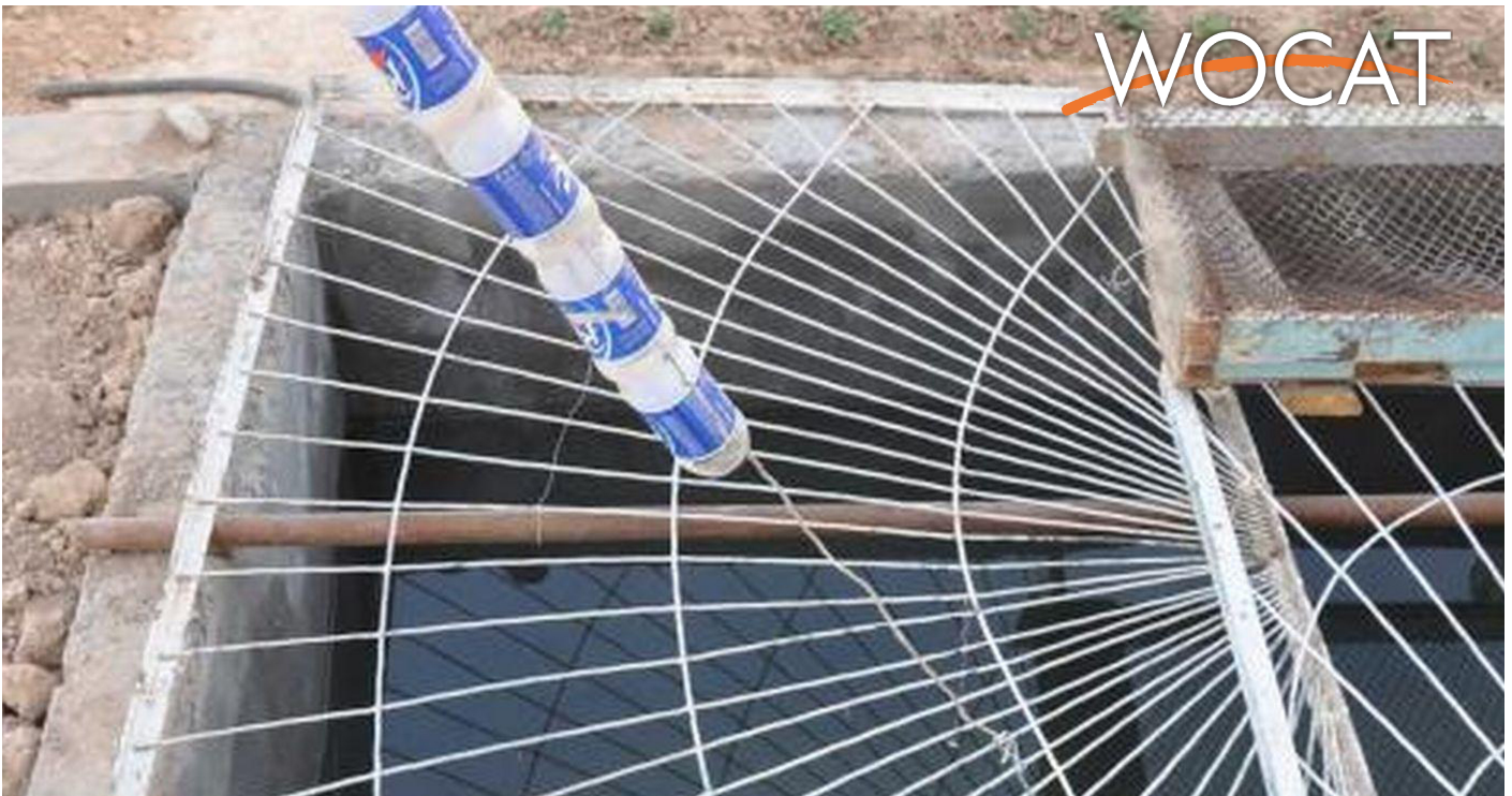
The plastic pipe running from the roof to the concrete tank. (S. Stevenson (Camp kuhiston))
