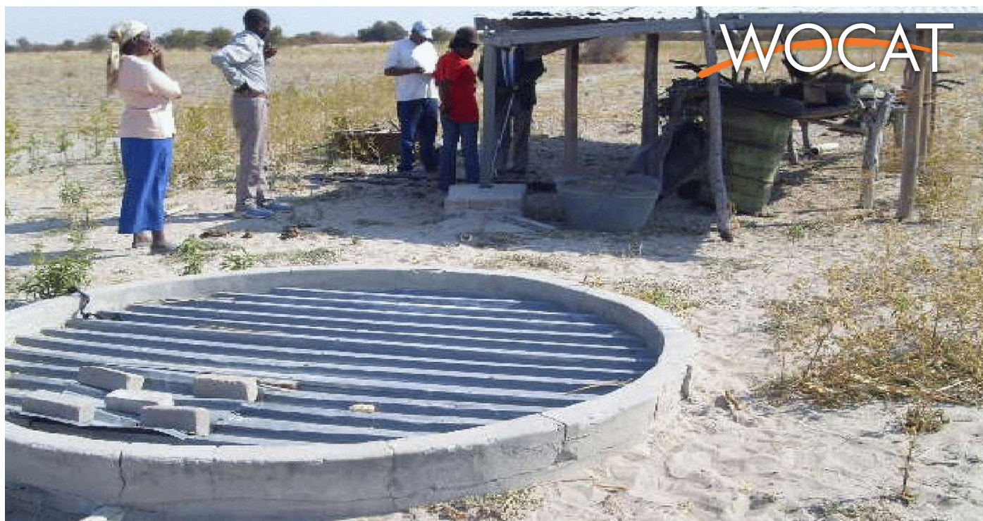
View of roof rainwater system at the lands in Mokoboxhane (J. Atlhopheng)
