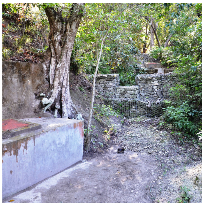
Physical protection of a water intake point
