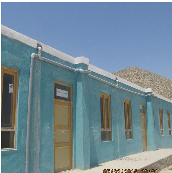
An overview of the pipe scheme of the roof rain water harvesting, Alik elementary school, Kishendeh (Saboor Popal (People In Need))
