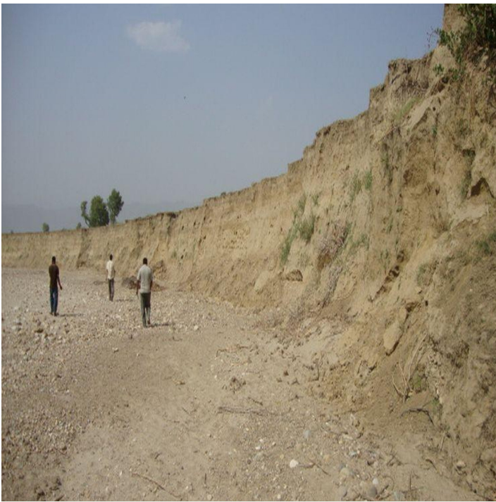
An eroded riverbank in Dang District (Udhaw Ghimire)
