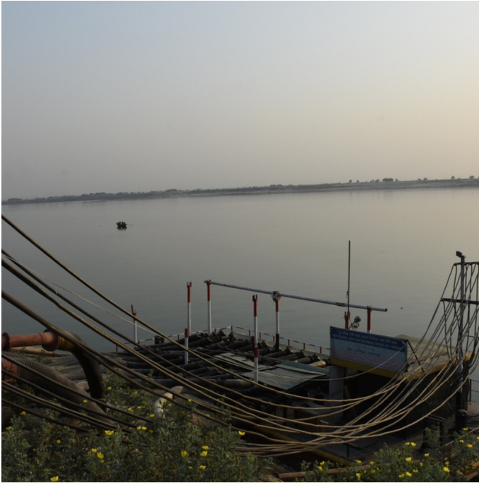
Pontoon with pumps at Padma river; there are 12 pumps operating (Zillul Bari)
